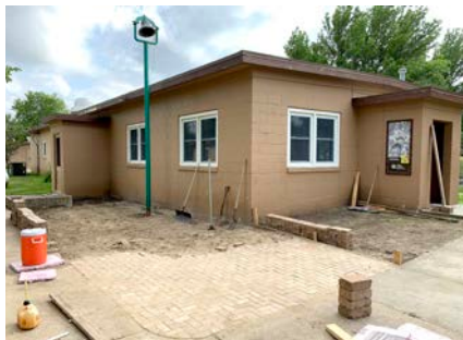
A concrete ramp and patios are being formed, poured and laid around the dining hall.
